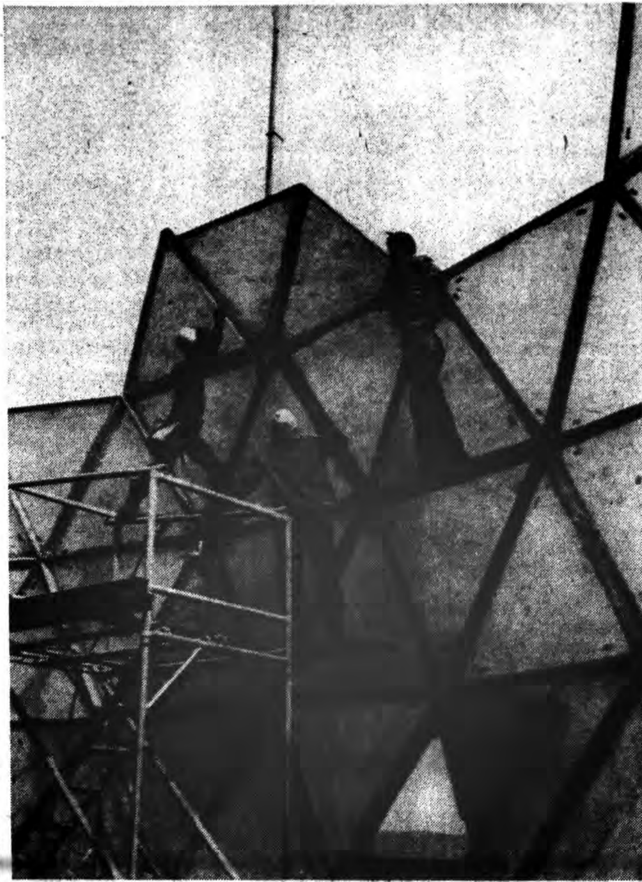
TOUGH JOB IN HIGH WIND —Three employees of the Roadmaster Construction Company, Saratoga Springs, finds assembly of the plastic sections of a radar dome a bit difficult in yesterday's high wind. They are constructing a new sectional plastic dome over a new and bigger radar "tail" in one of the towers at the Saratoga Springs Air Force Station.
